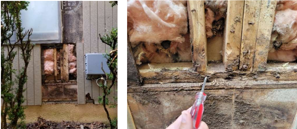
Photos 7 & 8: Deteriorated wood framing at base of wall, below window.
